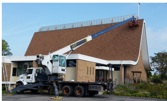
Roof repair work being done at the beginning of September by Mint Roofing.
